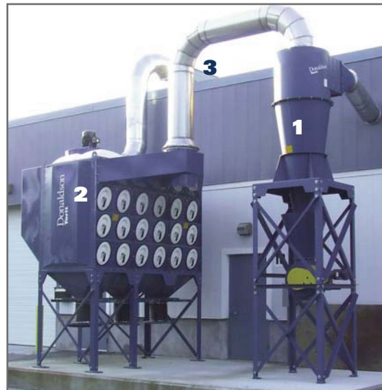
The new state-of-the-art spray booths at Falmer Thermal Spray (Salem, MA) are ducted outside the building into a (1) Donaldson® Torit® cyclone pre-cleaner, (2) then into Downflo® Oval (DFO) dust collector with Ultra-Web® filters, and (3) finally through a HEPA filter at the outlet on the roof. The system filters hexavalent chromium and other thermal spray particulate from the daily operations.
